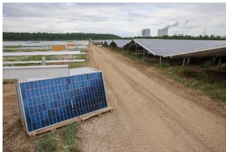
A solar farm is being constructed in Saxony, Germany, using 1.1 million solar modules imported from China (Image: Jan Woitas / Alamy)
